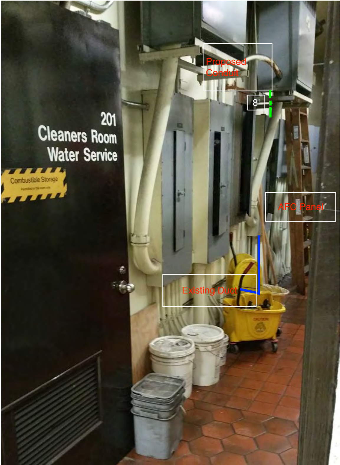
Photo #5: Existing Duct and Proposed Conduit feeding AFC panel SEMA in room 201
